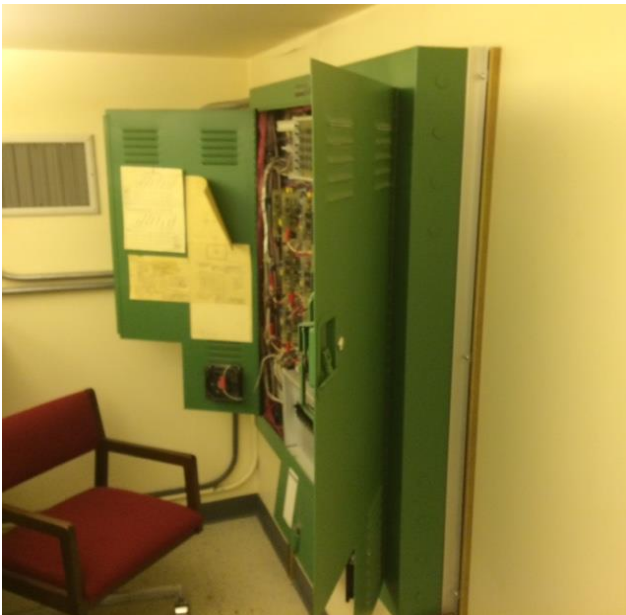
Existing Control panel
